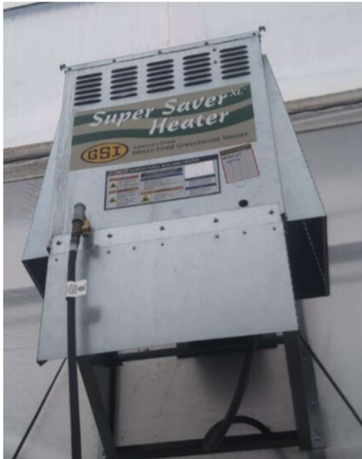
Figure 7: Greenhouse heating unit.
