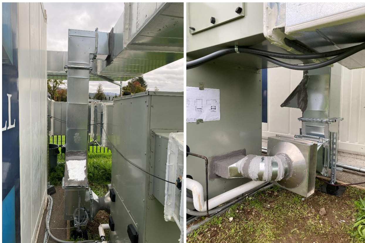
Figure 10: Partial heat exchanger bypass return duct connection with damper (left) and AHU connection with filter box (right).
