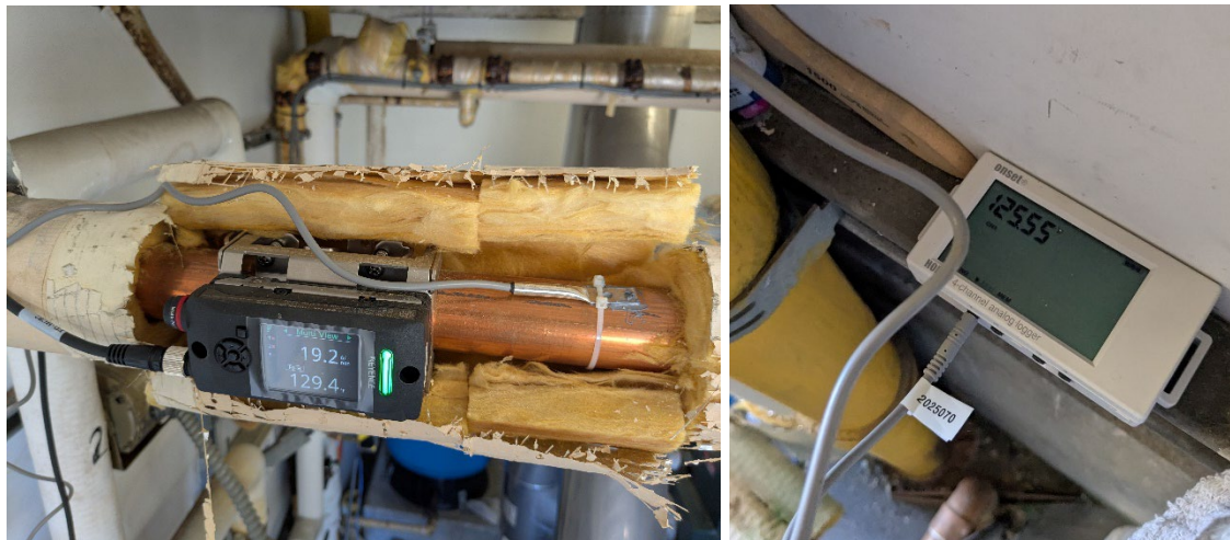
Figure 10: Flow meter and return water temperature sensor installation (left) with temperature logger (right).
