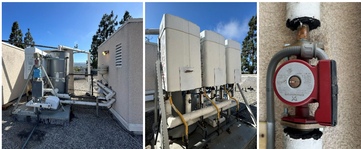
Figure 7: Site 4 hot water system, water heaters, and recirculation pump.
