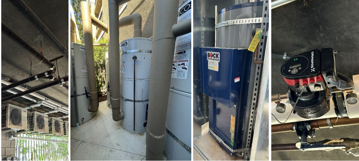
Figure 6: Site 3 HPWHs, storage tanks, swing tank, and recirculation pump.
