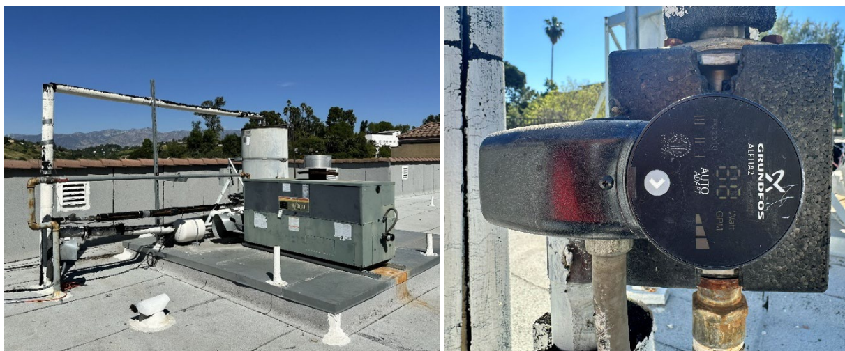
Figure 8: Site 5 DHW system and recirculation pump.
