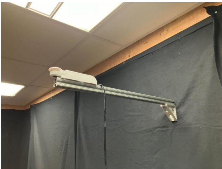
Figure 10: Control system illuminance sensor.
