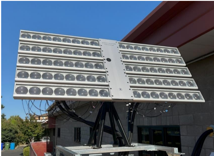
Figure 1: STF fiber optic daylighting system, fully installed.
