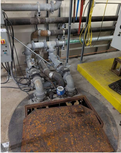
Figure 24: Hospital B sanitary pipe and tank.
