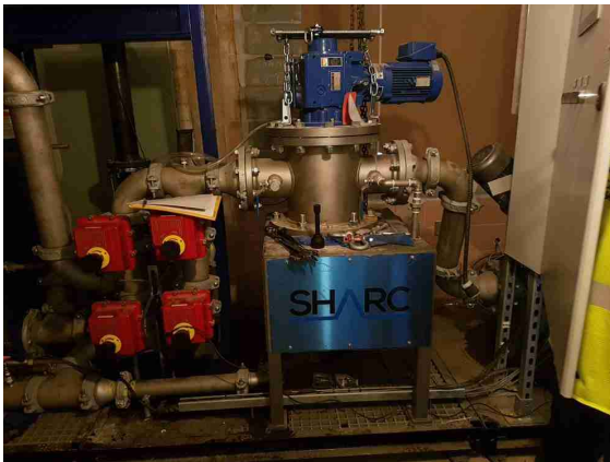
Figure 13: WET infrastructure at D.C. Water Administrative Building.
