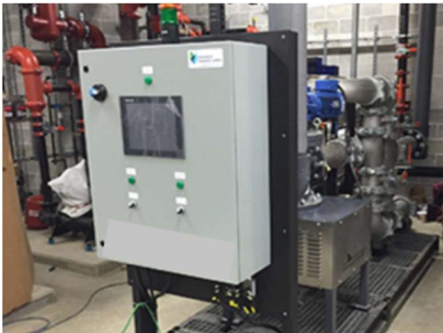
Figure 18: WET Infrastructure for Regional Water Resource Centre
