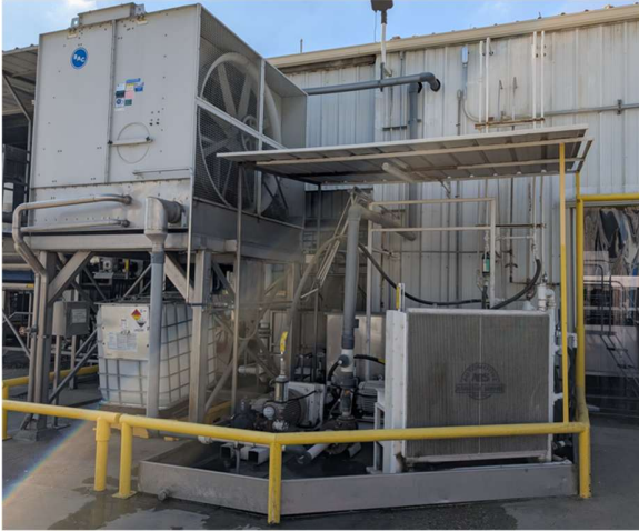
Figure 25: Cooling tower area for Food Processing Facility A.
