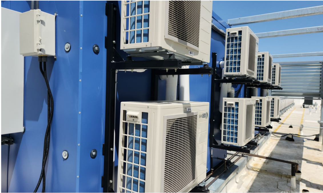
Figure 3: Packaged CHPWHs on rooftop.
