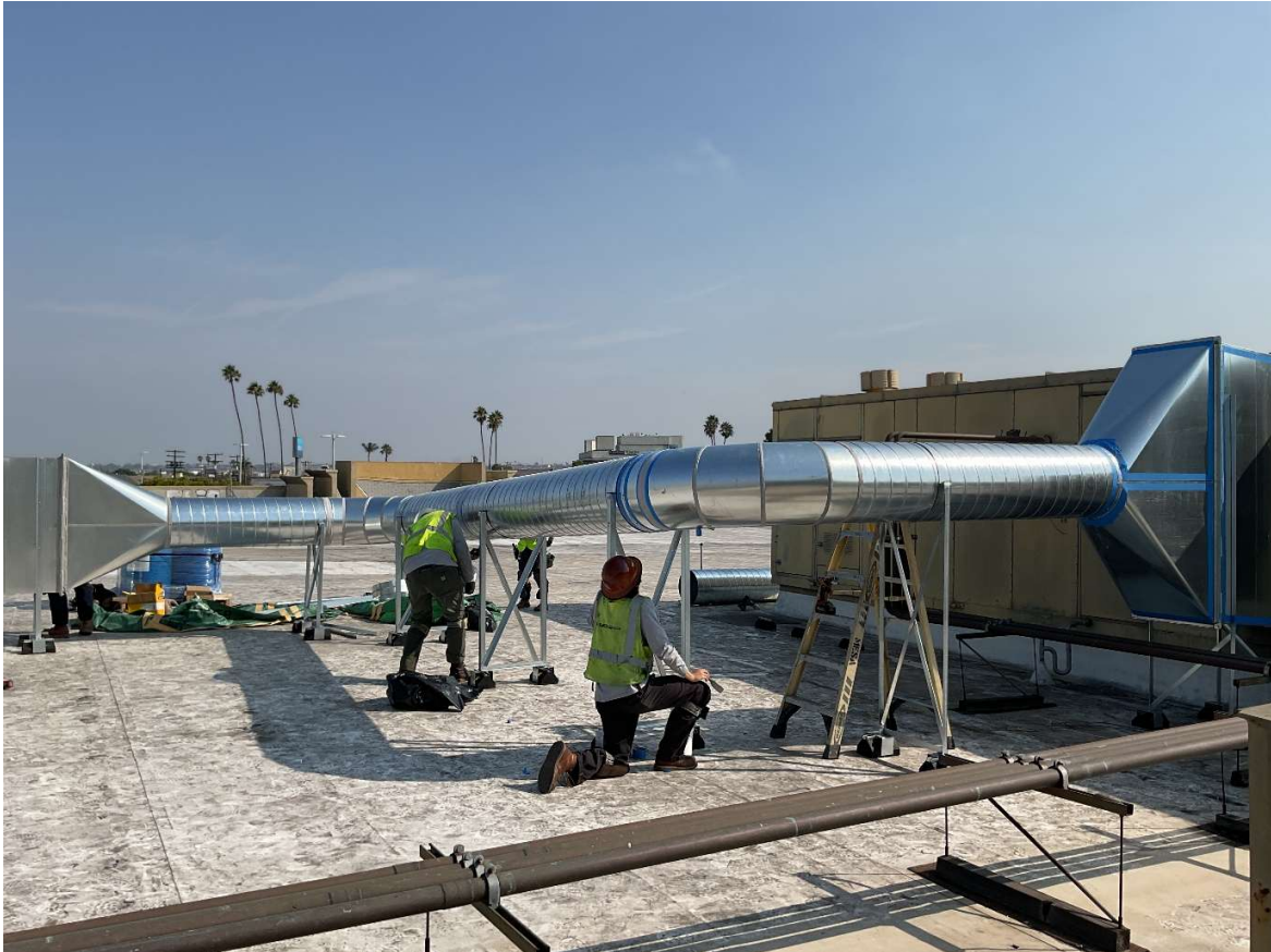
Figure 5: ES-LD-DOAS piping to existing rooftop air handler.
