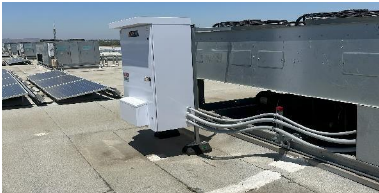
Figure 23: CU5E compressor with the ET.
