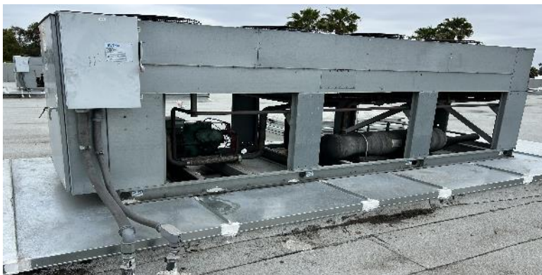
Figure 7: CU4 condensing unit.
