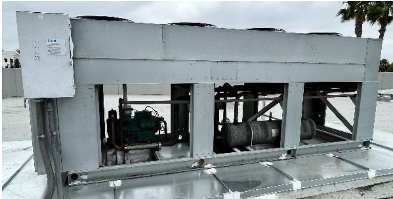
Figure 6: CU3 condensing unit.
