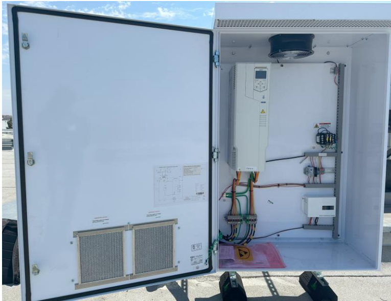
Figure 13: Inside view of the ET.
