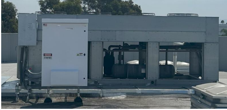
Figure 14: CU3 condensing unit with the ET.
