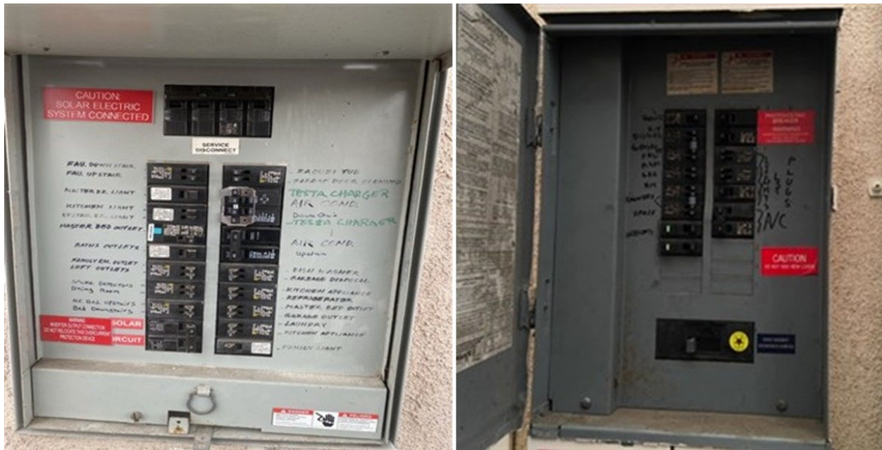
Figure 18: Examples of electrical panel upgrade (left) and optimization (right) opportunities.
