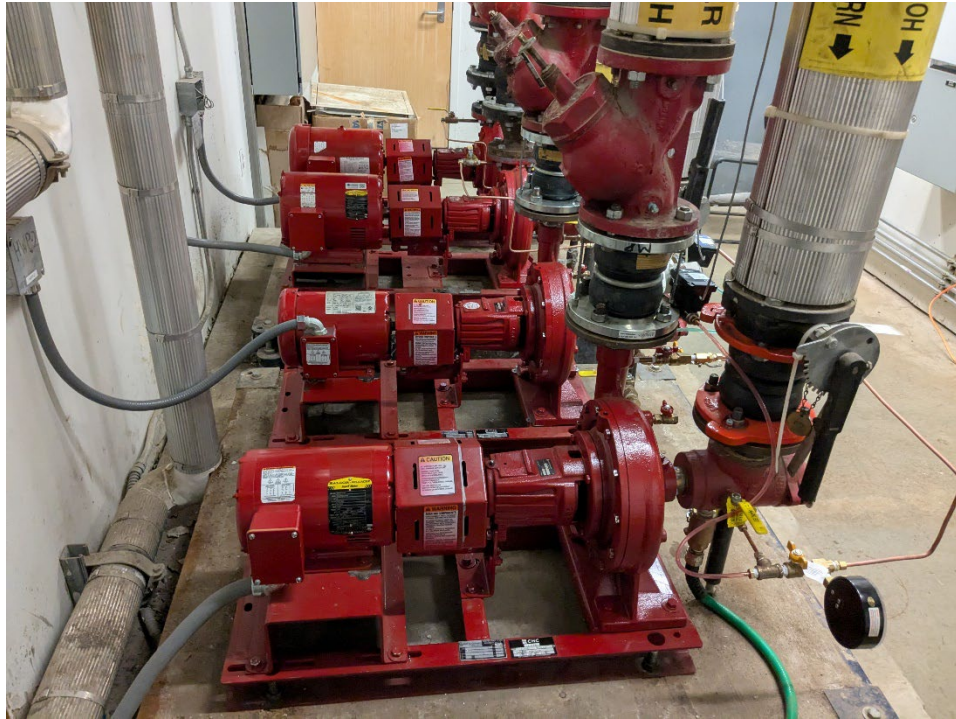
Figure 7: Four pumps after final installation. The manufacturer painted all motors red as is typical for their products.
