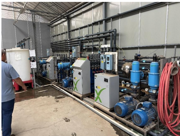
Figure 68: Irrigation and fertigation systems serving Greenhouse F.
