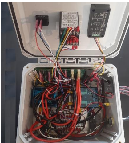
Figure 5: HCC internal wiring.
