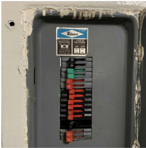
Electrical Panel label photo example
