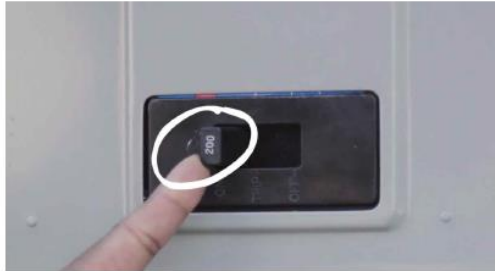
'Main circuit breaker' or 'main breaker'
