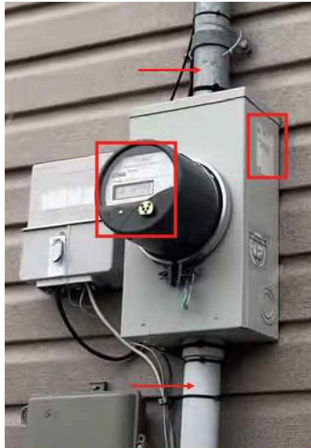
Electrical meter, meter labels, incoming pipe, and outgoing pipe
