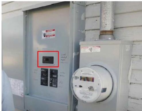
Main breaker next to electrical meter
