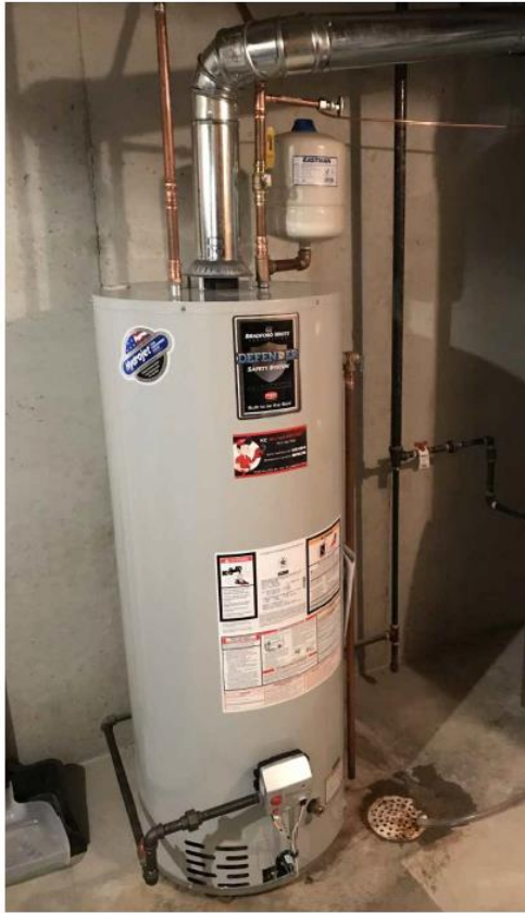
Storage Tank - Gas water heater
