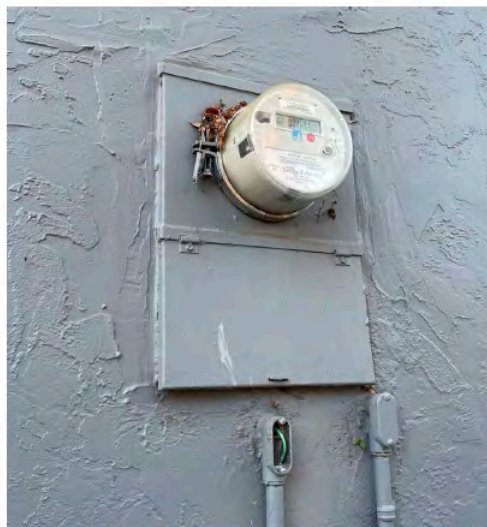
Pipes are not visible as they are inside the wall
