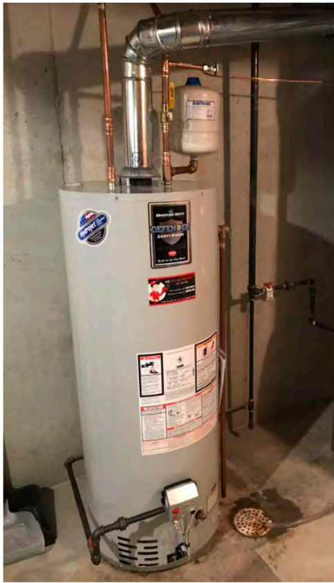
Storage Tank - Gas water heater
