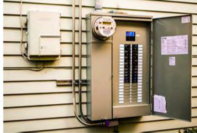
Circuit Breakers photo example
