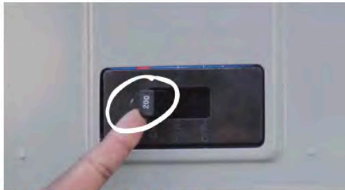
'Main circuit breaker' or 'main breaker'
