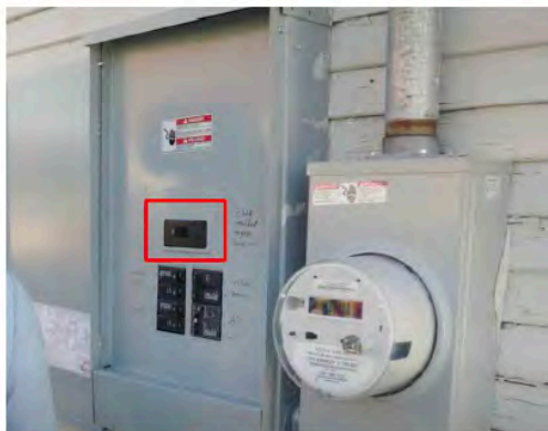
Main breaker next to electrical meter
