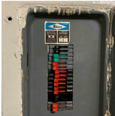
Electrical Panel label photo example
