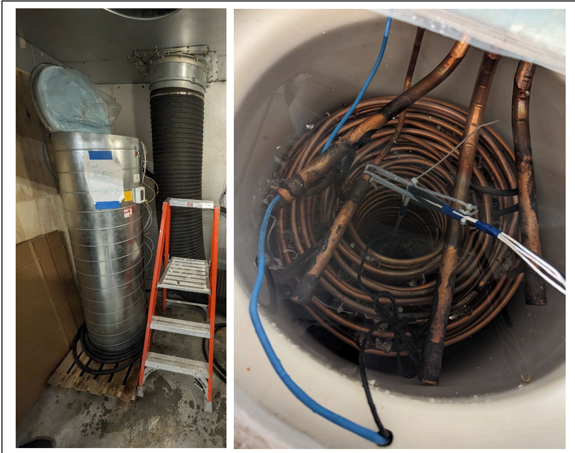
Figure 5. WT of the MFHP manufacturer system installed in the WCEC indoor chamber (left). WT refrigerant-to-water and water-to-water heat exchangers with temperature sensors (right).
