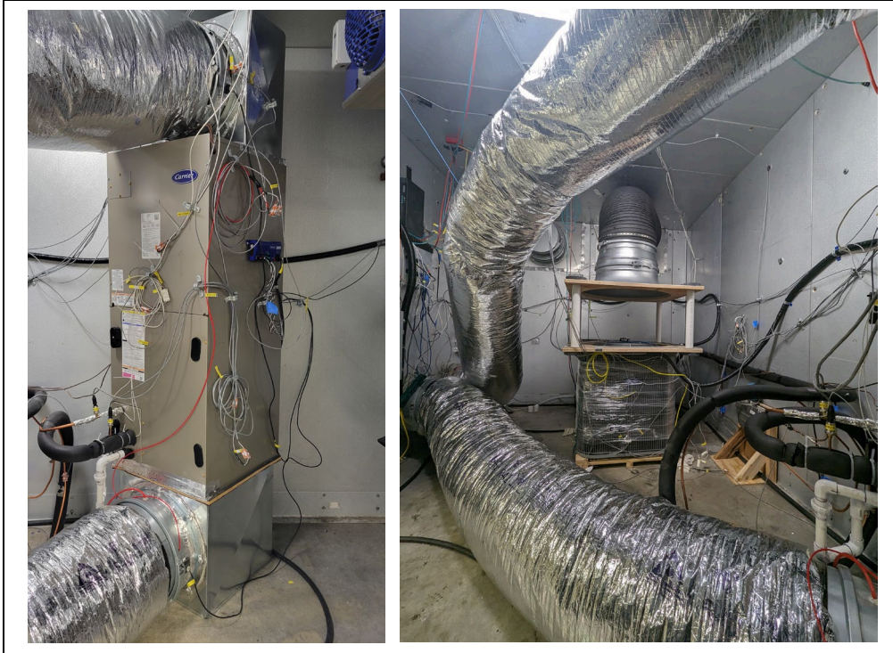
Figure 4. AHU instrumented and ducted (left). MFHP ODU instrumented and exhaust duct connected with a stand-off (right).
