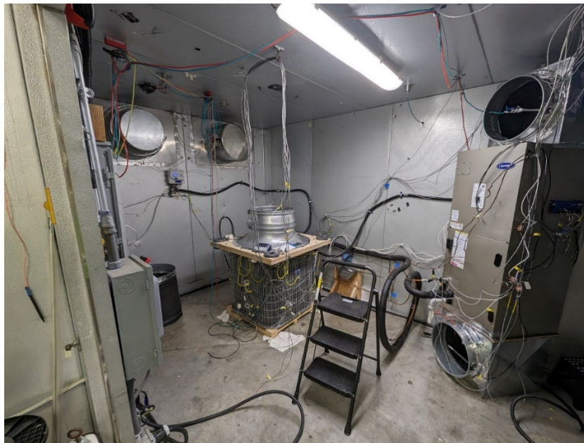
Figure 3. MFHP ODU and AHU being installed and instrumented in the outdoor chamber.
