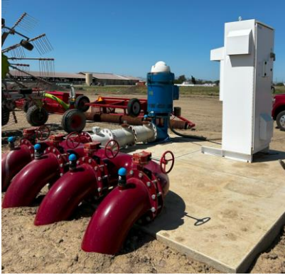
Figure 18: Irrigation well #1 groundwater pump.
