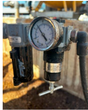
Figure 32: Pressure gauge for filter.
