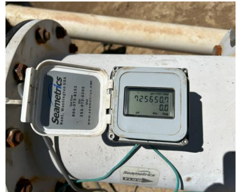
Figure 28: Wastewater pump #2 flowmeter.
