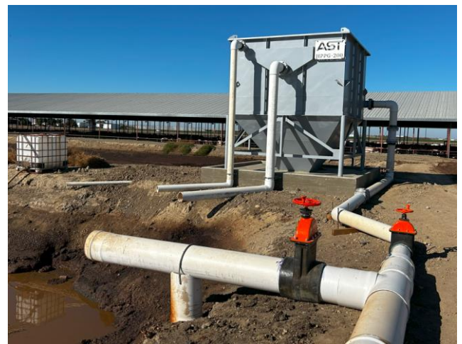
Figure 37: Floating bead filter, rear view.
