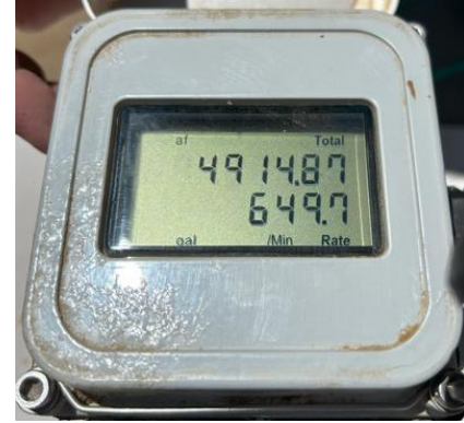
Figure 20: Irrigation well #1 flowmeter.
