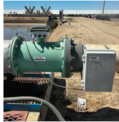
Figure 24: Wastewater pump #1 flowmeter.
