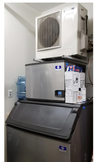
HP Mounted Near Ceiling. (Croton100 2020)
