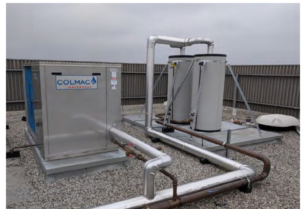
Colmac Split HPWH System with Hot Water Storage Rooftop Installation
