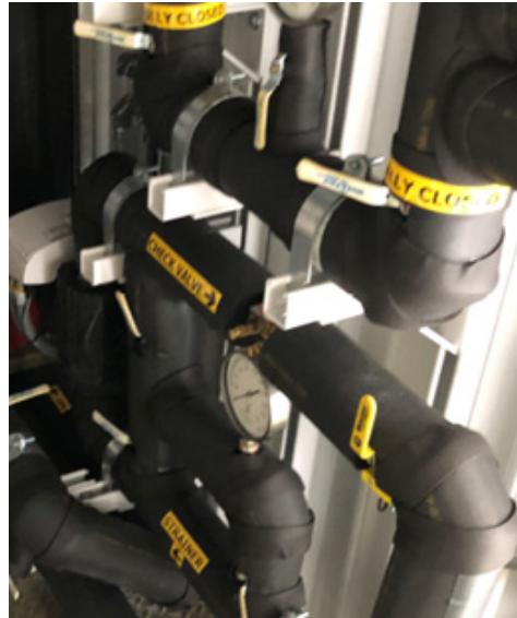
Continuous Pipe Insulation with External Pipe Supports. (Ecotope 2021)
