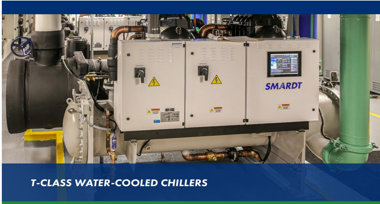
Figure 6: Smartd Oil free water cooled chillers
