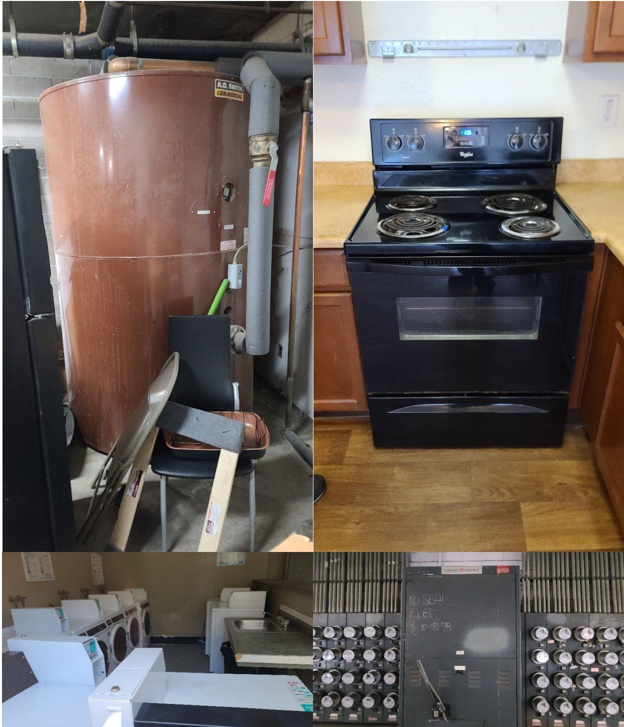
Top row, left to right: 1600A main breaker and dedicated transformer pad. Second row, left to right: central DHW and in-unit electric cooking range. Third (bottom) row: common area laundry and meter bank.
