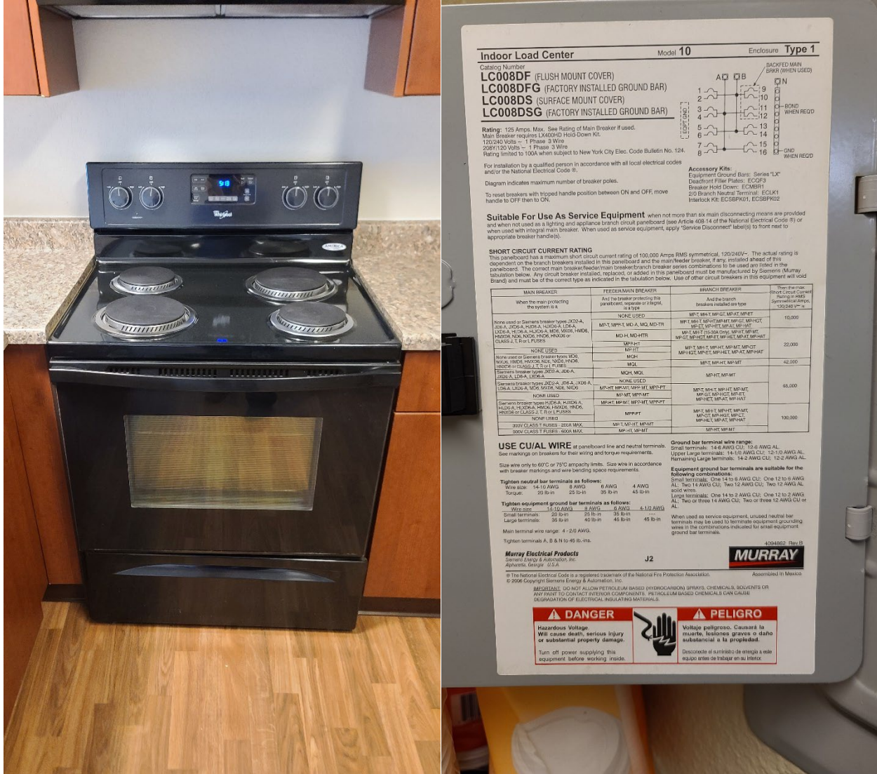
Top row, left to right: unit main breaker and meter bank. Second row, left to right: heat pump located on outside of building and DHW. Third (bottom) row, left to right: in-unit electric cooking range and unit breaker panel.
