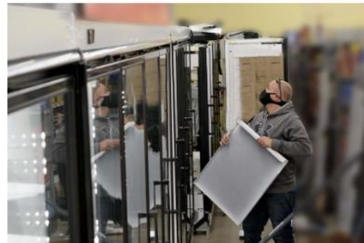
FEWER WORKERS: The entire labor force is smaller than it used to be pre-pandemic, but the issue is even more severe in construction. (Courtesy of Professional HVAC/R Services Inc.)
